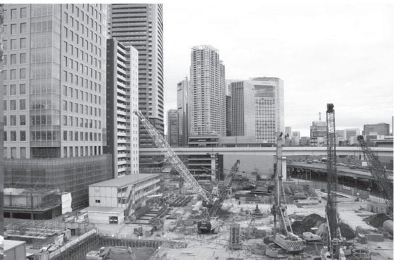
Construction site in Shiodome, the new cluster of office and residential towers in Chuo ward.
